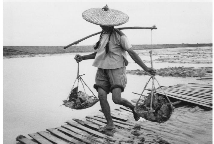
Chinese worker brings dirt to a pond levee being built, Guangdong Province coastline of the South China Sea.
